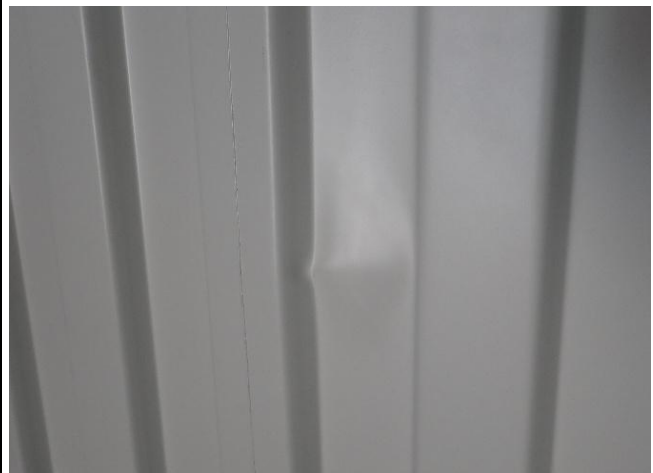
8. Other view front panel conditions.
