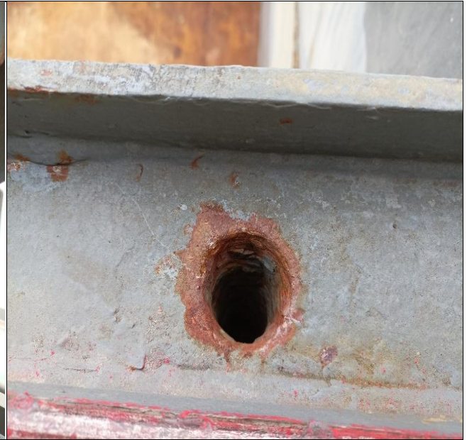
13. Hold Nr. 2, drain hole conditions.
