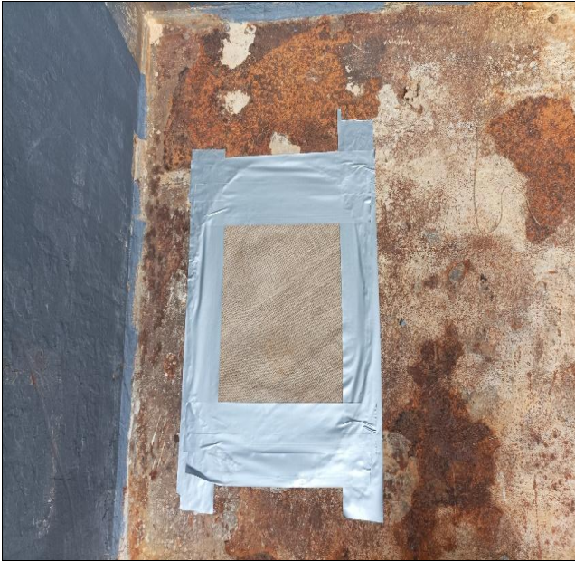
8. Hold Nr. 2, bilge/Pe covered with burlap and sealed with tape.
