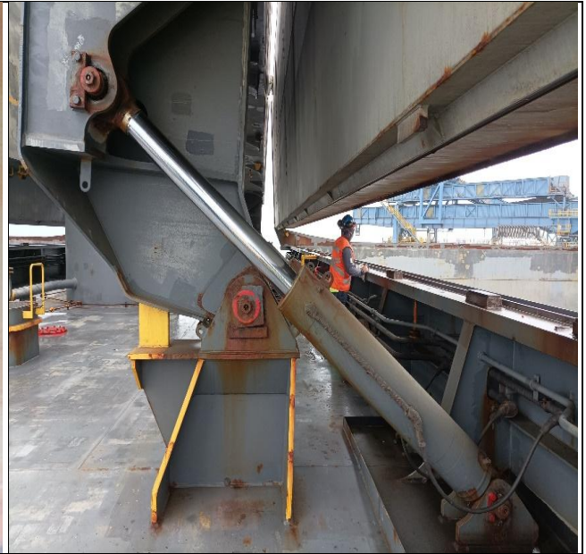
17. Hold Nr. 2, hydraulic system without leaking.
