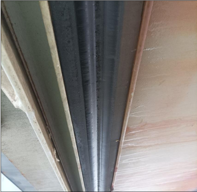
16. Hatch cover hold Nr. 2, rubber packing condition.
