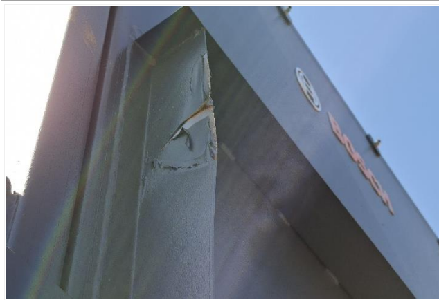
3. External frame dented, scratched and rusty.
