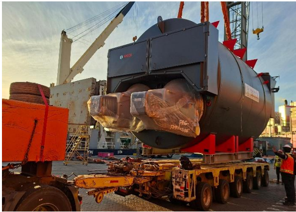
21. Boiler during discharge operation
