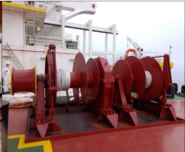
22.View of Ss, Aft, winch.
