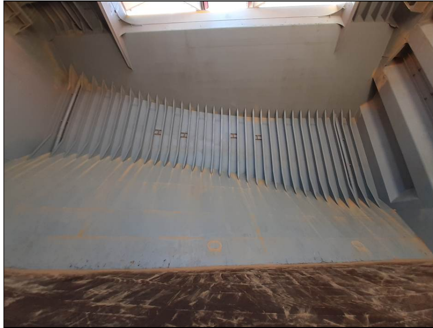
31. Side/shell plating Ss with paint scratched.
