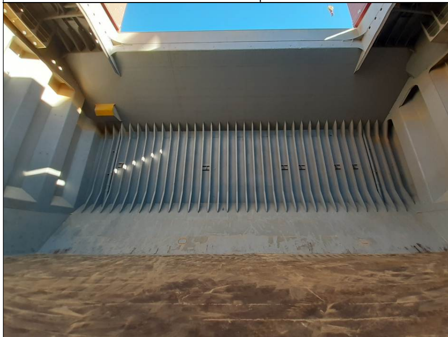
58. Side/shell plating Ps, with paint scratched and rust.
