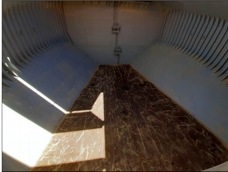
27. General view of C/H N°1.
