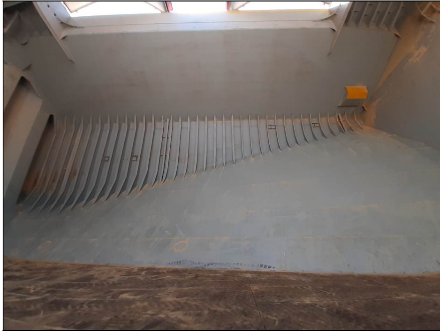
69. Side/shell plating Ss, with paint scratched and rust.
