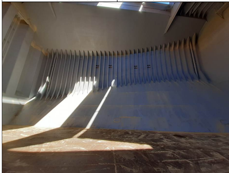
30. Side/shell plating Ps with paint scratched.
