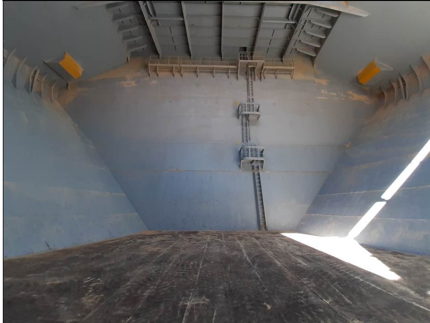
67. Aft bulkhead with paint scratched.
