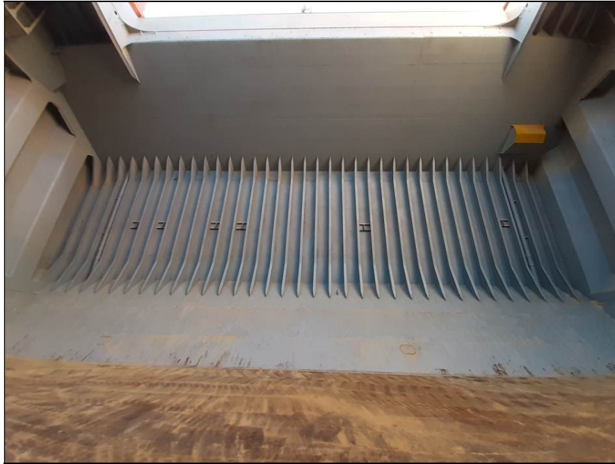
59. Side/shell plating Ss, with paint scratched and rust.
