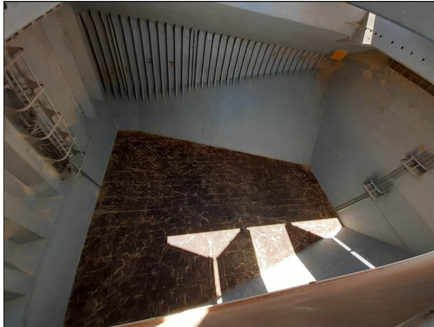
65. General view of C/H N° 5.
