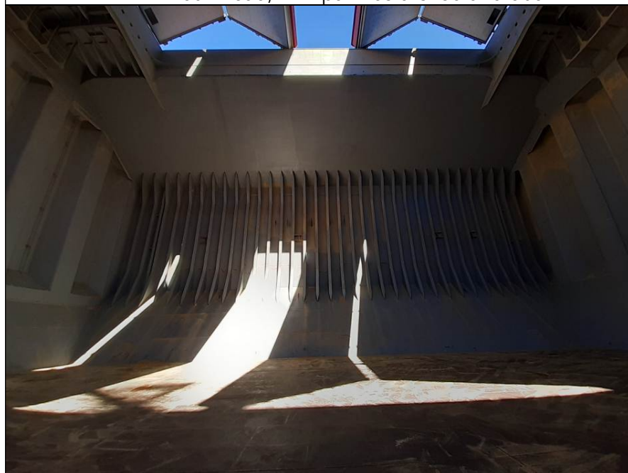
48. Side/shell plating Ps, with paint scratched.
