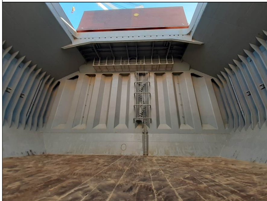
56. Fwd bulkhead with paint scratched.
