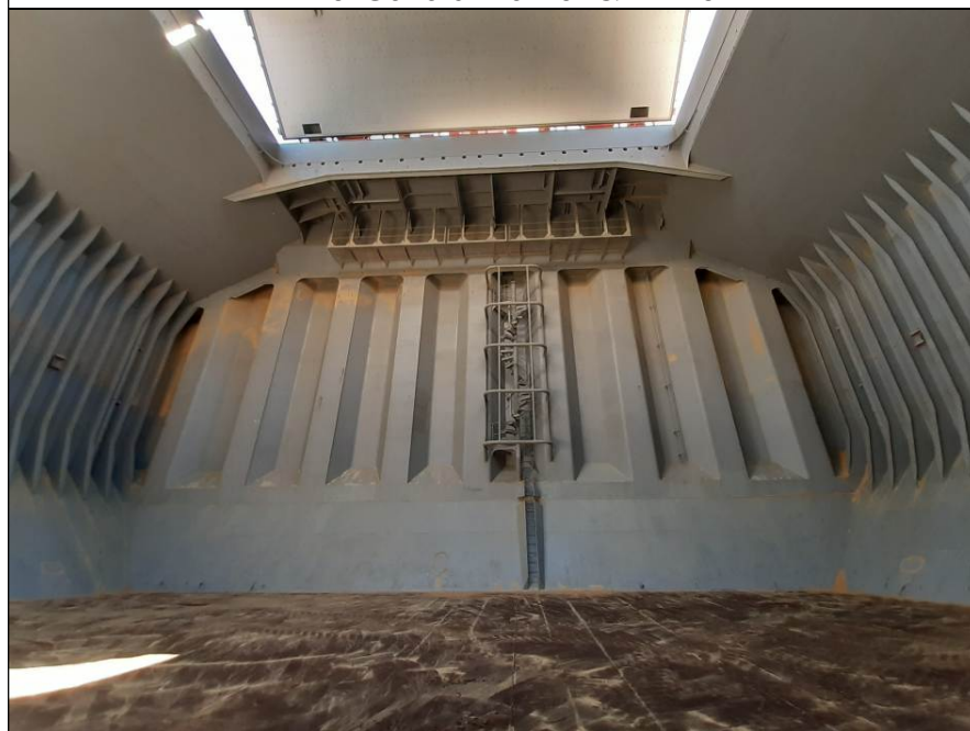
46. Fwd bulkhead, with paint scratched and dust.
