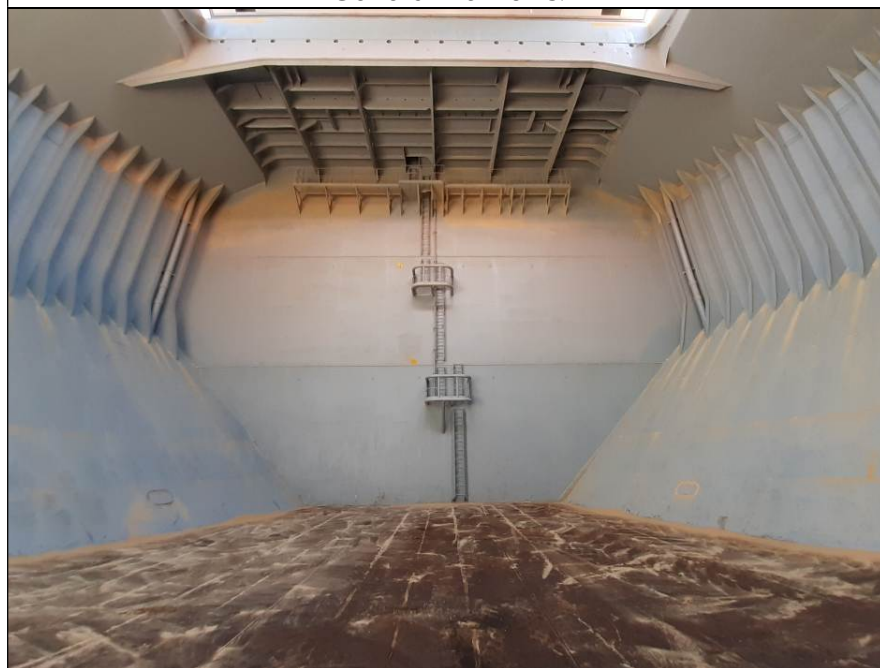
28. Fwd bulkhead with paint scratched and rust.
