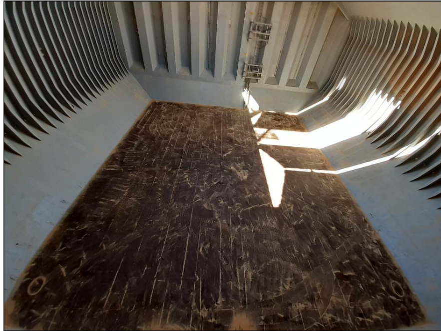
45. General view of C/H N° 3.
