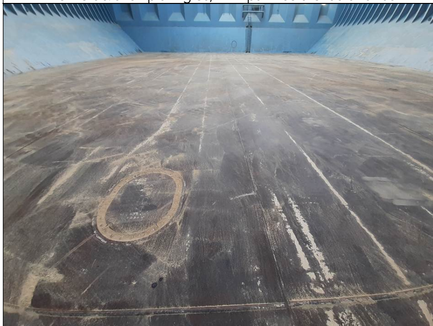
60. Tank top plating rusty.
