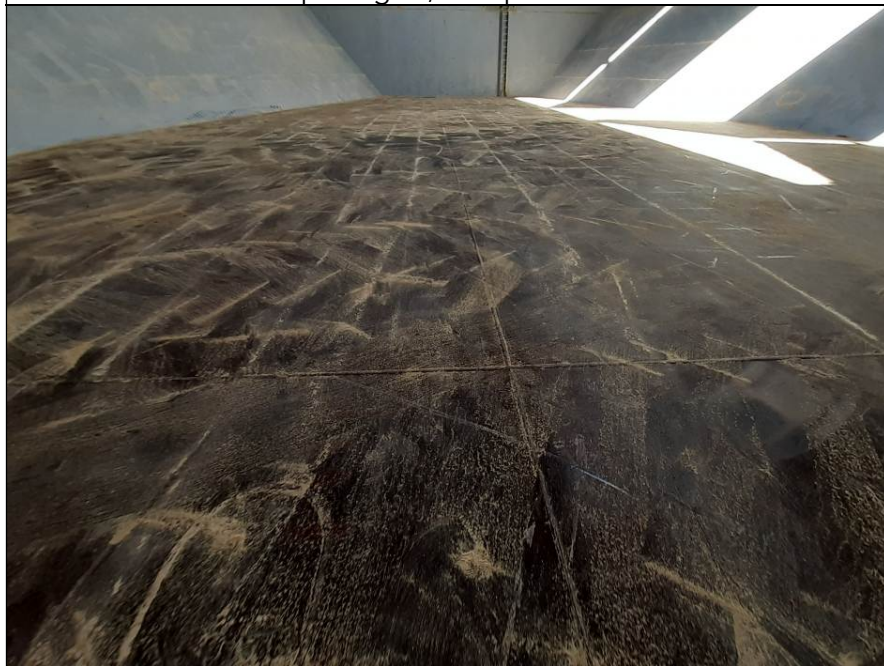
70. Tank top plating rusty, with dust of cargo discharged.
