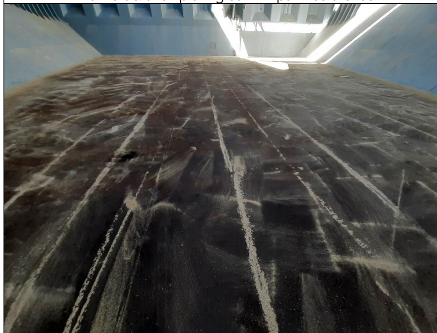
32. Tank top plating with dust.
