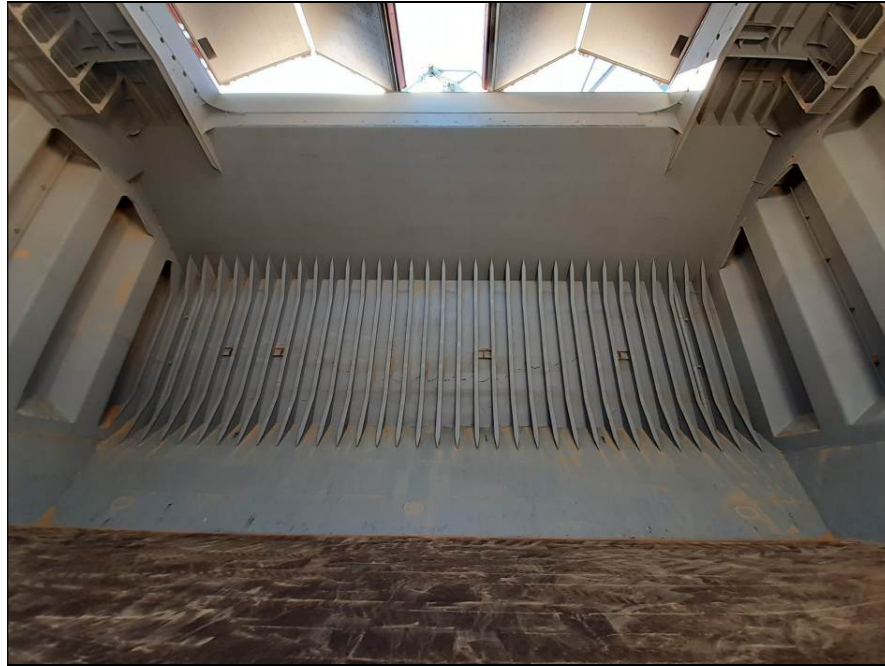
49. Side/shell plating Ss, with paint scratched and rust.
