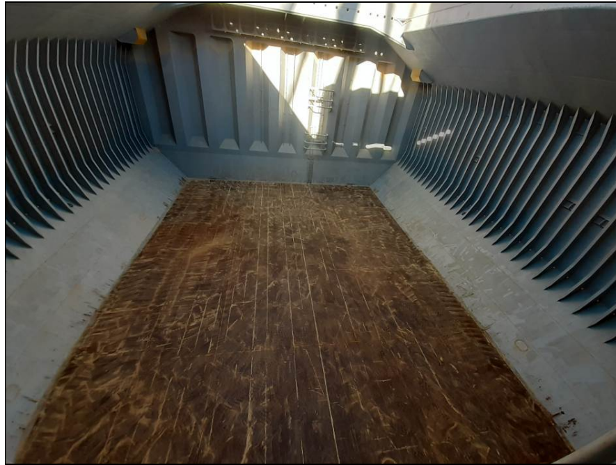
55. General view of C/H N° 4.
