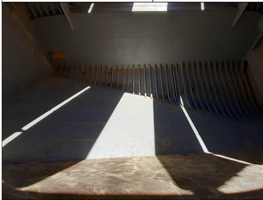
68. Side/shell plating Ps, with paint scratched and rust.
