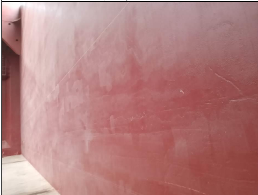
50. Side/shell plating Ps, with paint scratched and dust.
