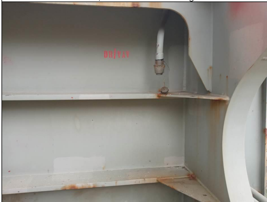
64. Hatchcover No. 4, non-return valves in good conditions.
