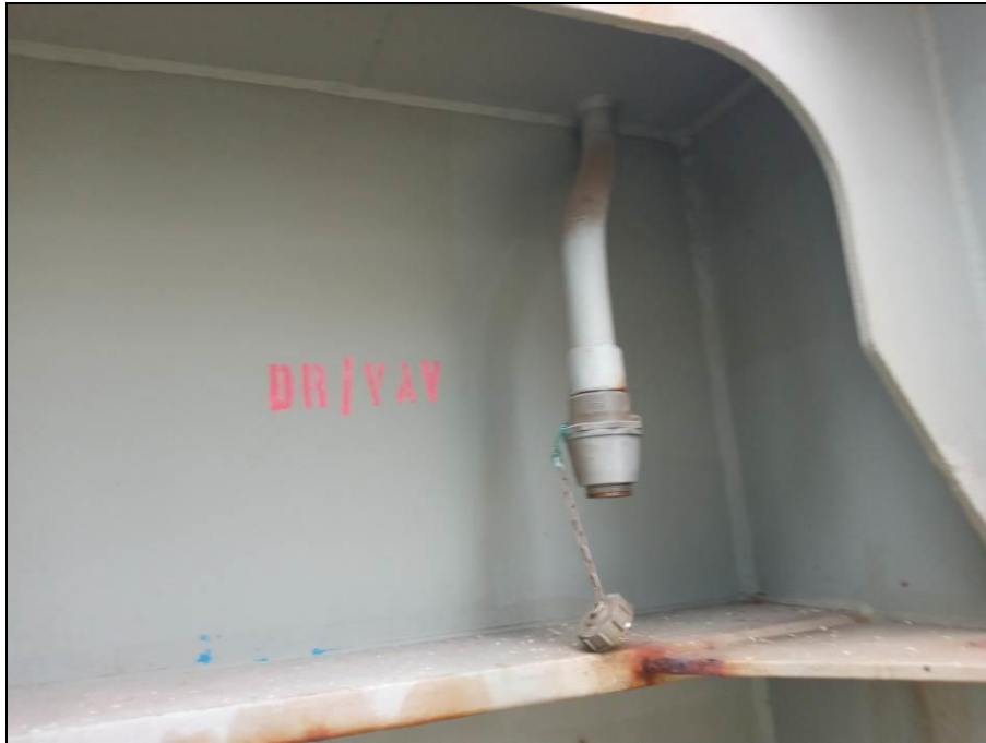
53. Hatchcover No. 3, non-return valves in good conditions.
