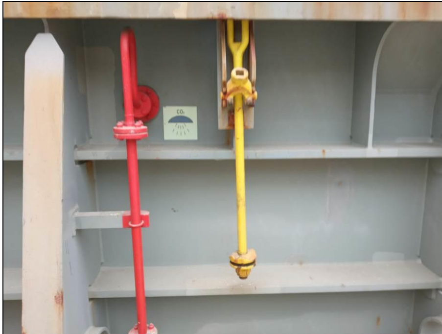
45. Hatchcover No. 2, active cleats in good conditions.
