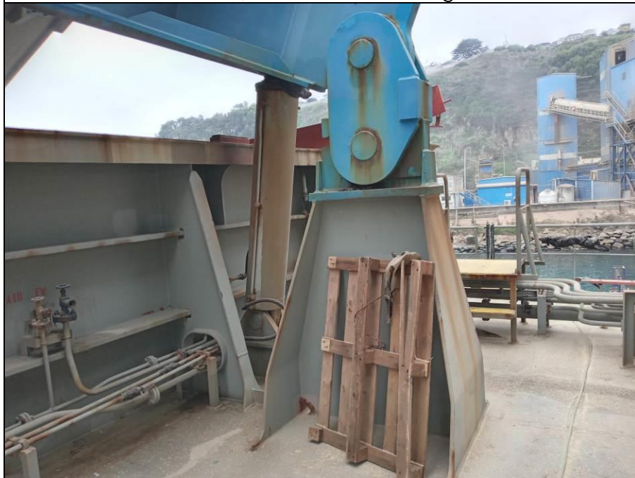
54. Hatchcover No. 3, hydraulic system in good conditions.
