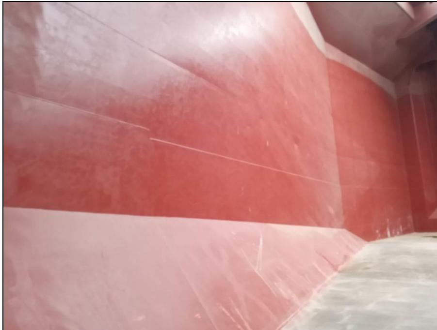
31. Side/shell plating Ss with paint scratched.
