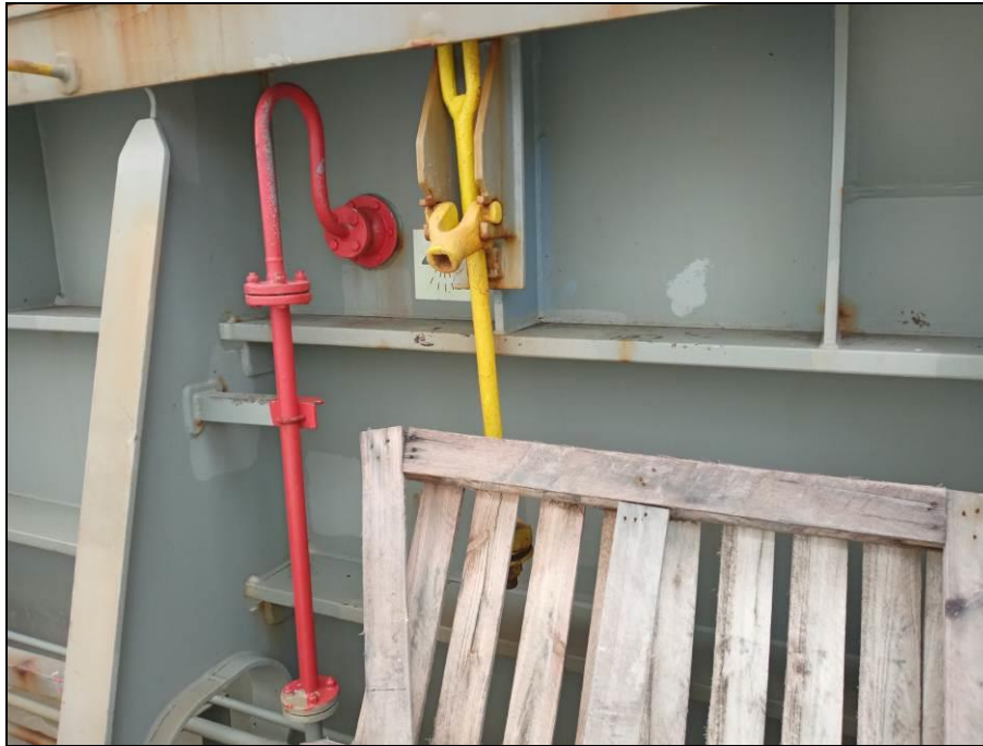
73. Hatchcover No. 5, active cleats in good conditions.
