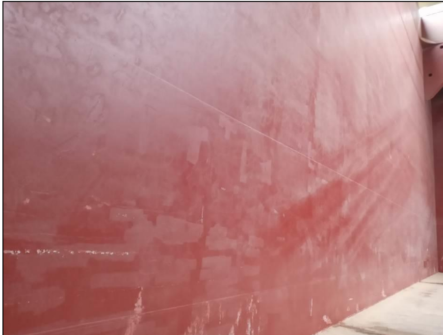
51. Side/shell plating Ss, with paint scratched and rust.
