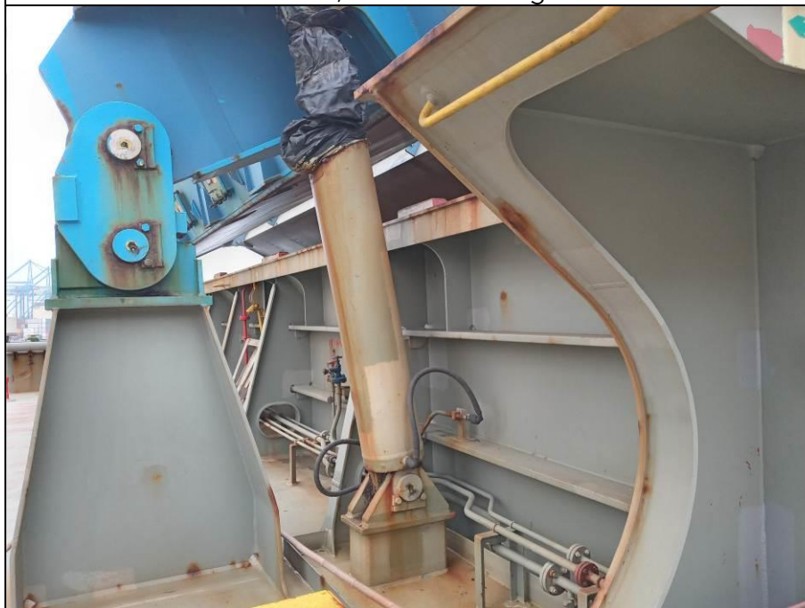
74. Hatchcover No. 5, hydraulic system in good conditions.
