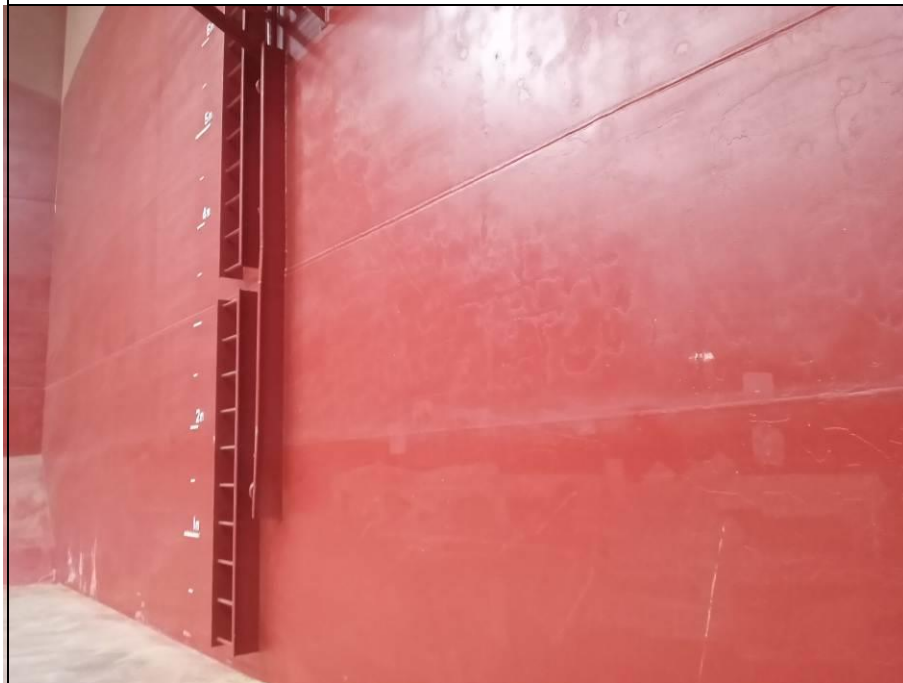
28. Fwd bulkhead with paint scratched.
