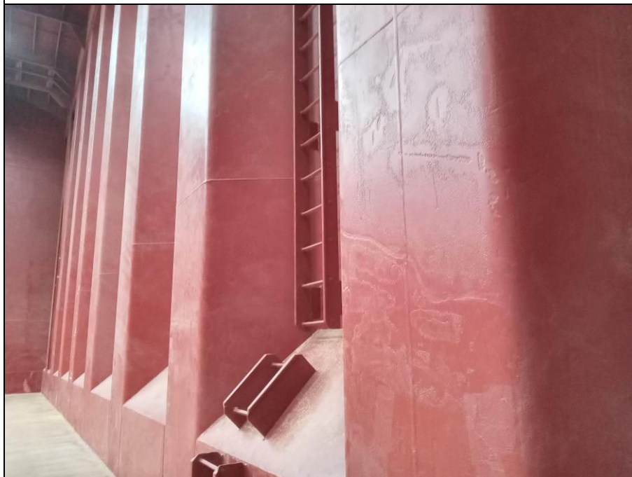
48. Fwd bulkhead, with paint scratched and dust.
