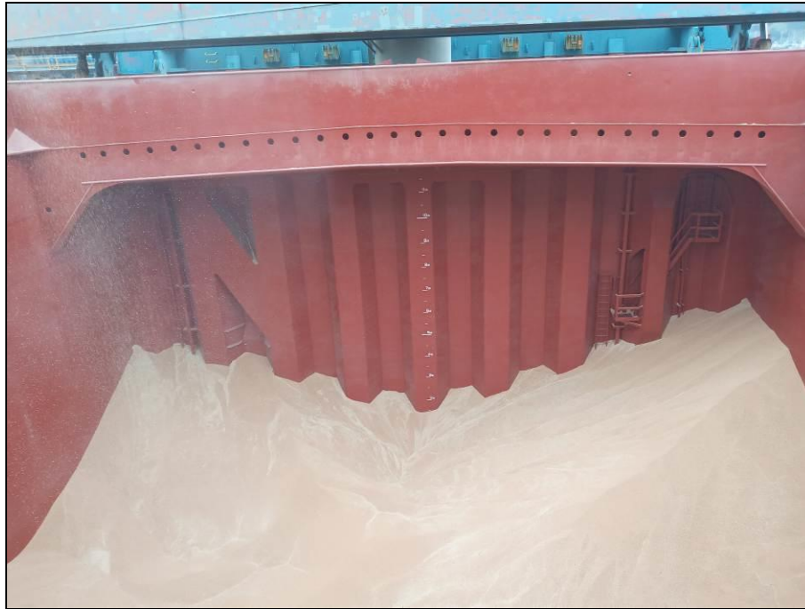
59. Aft bulkhead with paint scratched and rust.
