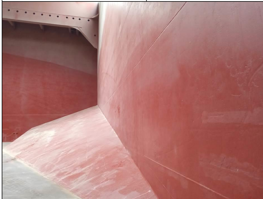
70. Side/shell plating Ps, with paint scratched and rust.
