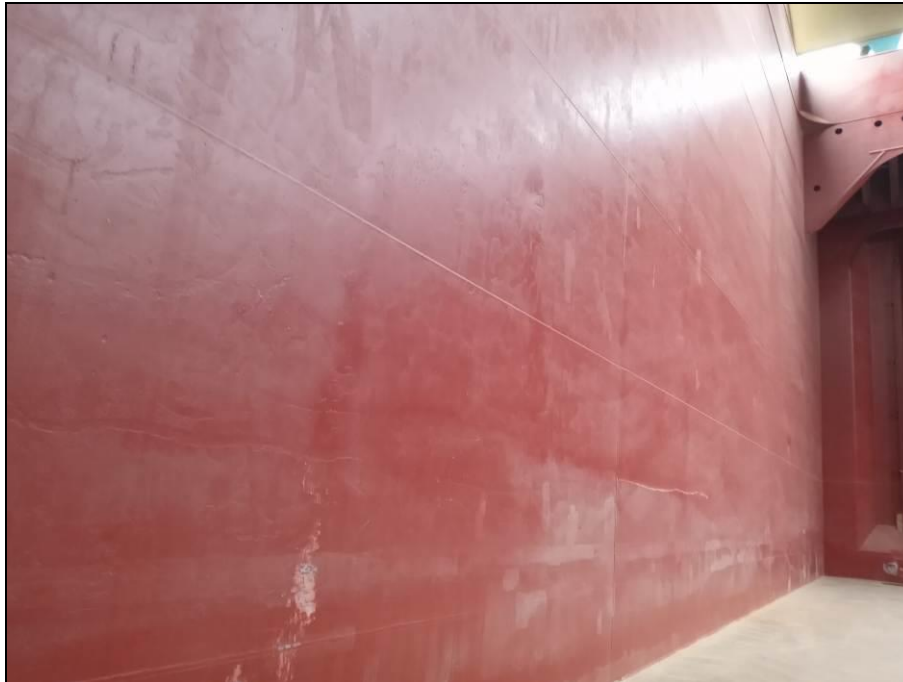
41. Side/shell plating Ss, with paint scratched and rust.
