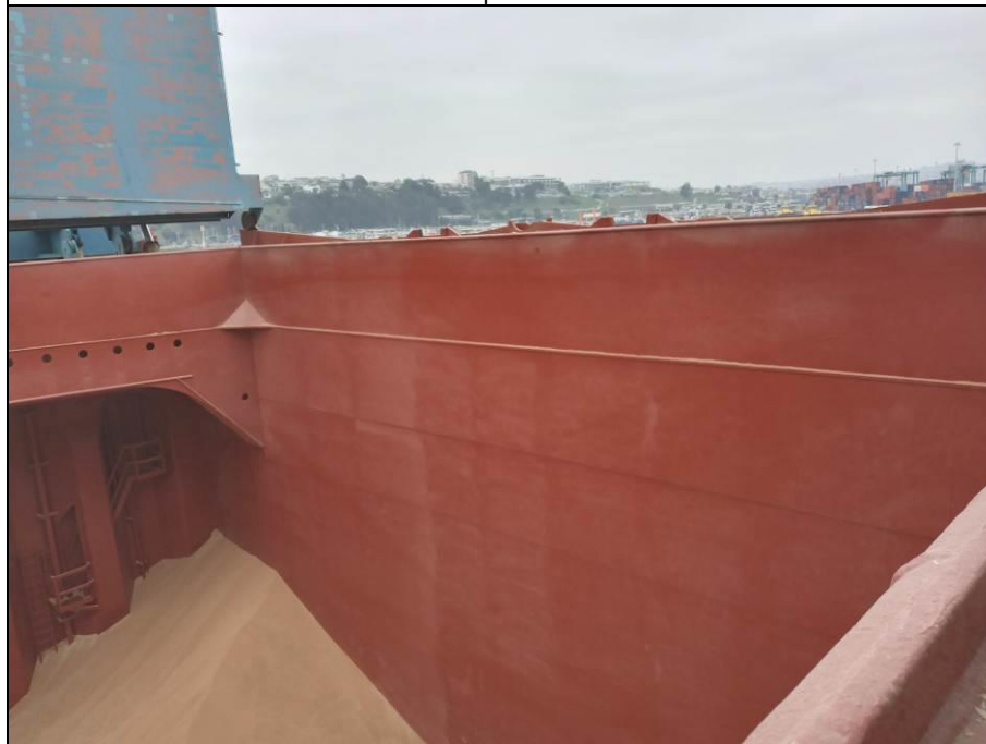
60. Side/shell plating Ps, with paint scratched and rust.
