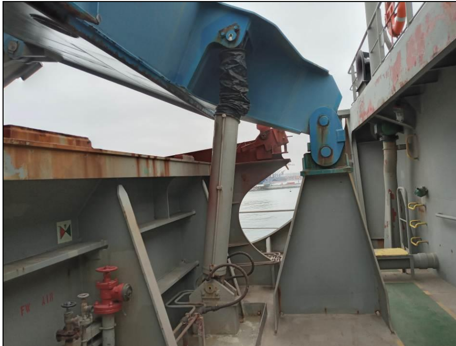
35. Hatchcover No. 1, hydraulic systems in good conditions
